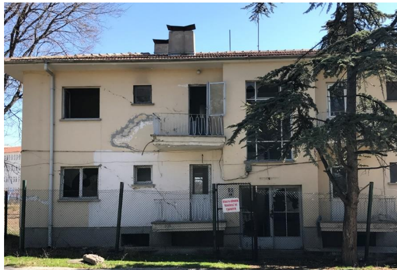
Figure 4.9. d-type housing evacuated due to danger of collapse (Author,2017)
