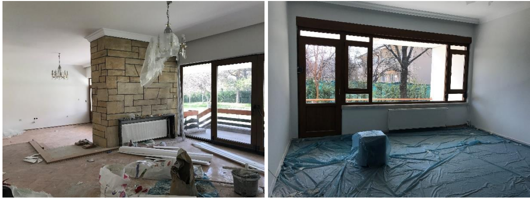
Figure 4.12. Renovation of floor tiles and joinery of lodgin of General Director of TSFAS
