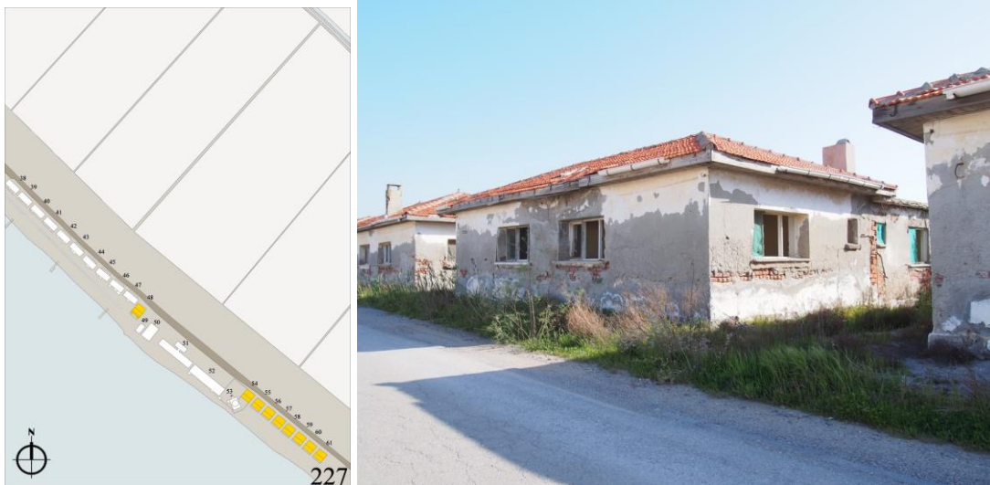
Figure 119 Site plan and the northern corner of the lodging type 6 (Author, April 2016)
