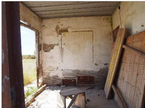
Room and closed window opening (3)
