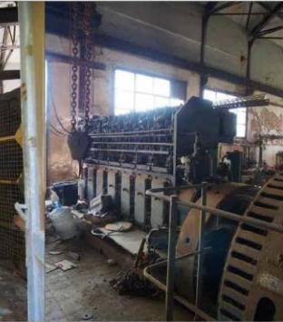
Power plant system (1)
