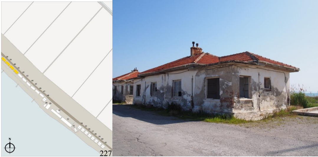
Figure 117 Site plan and the northern corner of the lodging type 4 (Author, April 2016)
