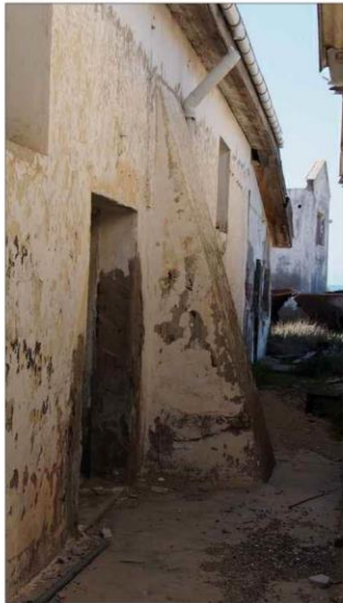
Only remaining buttress
