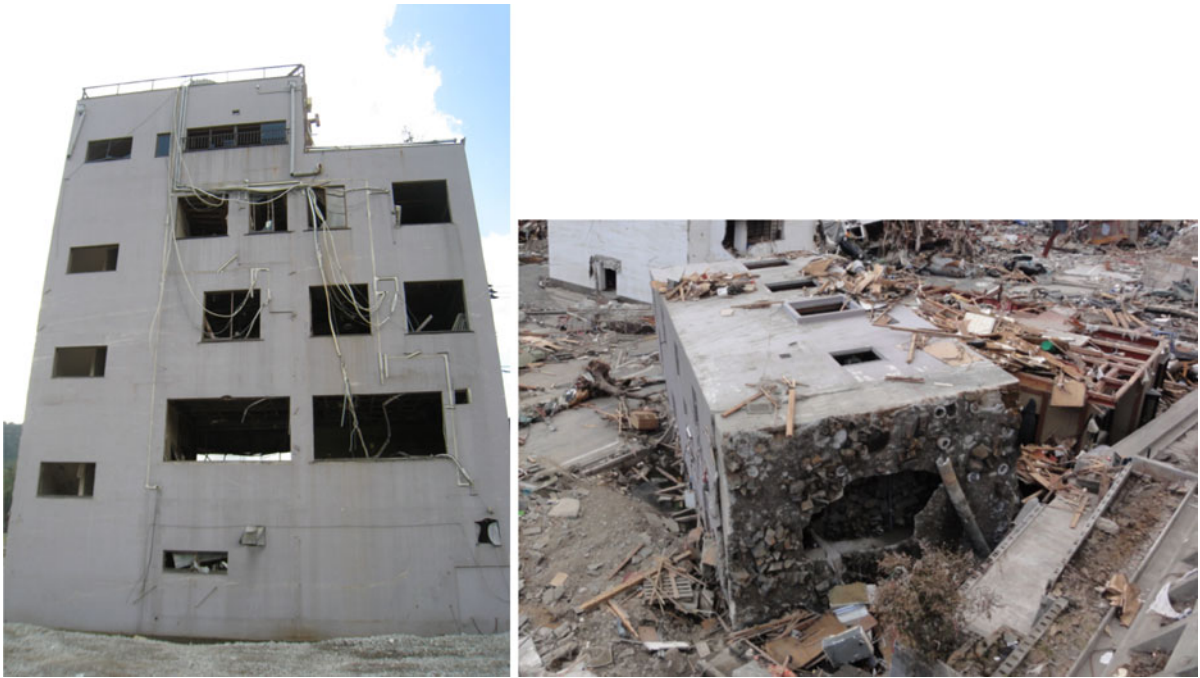
Figure 19 Building X (sea front), which survived (29/9/2011), and building B, which was overturned (29/3/2011)
