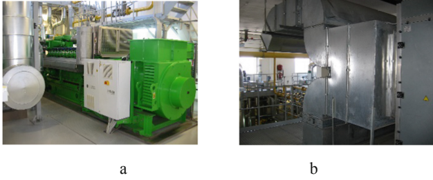
Fig. 1. Cogeneration gas engine module JMS GE Jenbacher (a) and waste heat recovery central conditioner for cooling engine room intake air (b)
