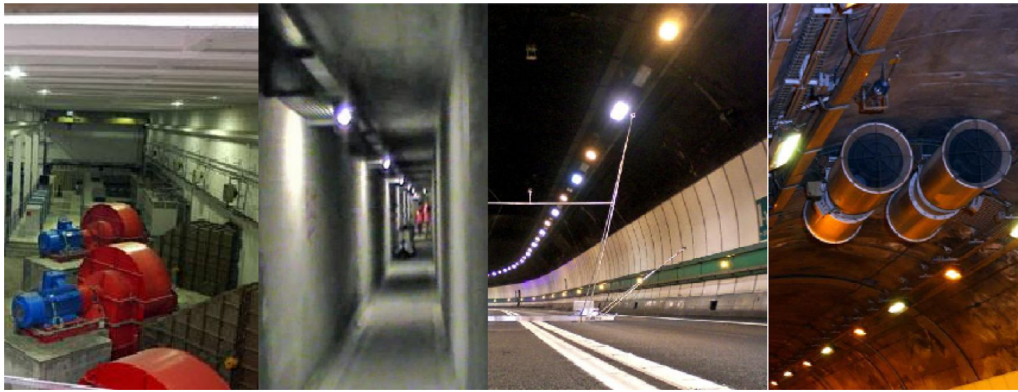
Fig. 2. Details of the Mont Blanc Tunnel ventilation system: (left to right) interior of the ventilation central on the Italian side; underground fresh air channel; fresh air supply vents along the walkside; a pair of jet fans.
