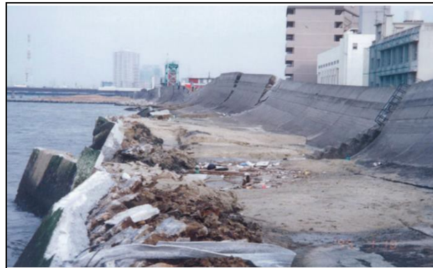
Fig. 7 - Slides due to earthquake triggered soil liquefaction at the Yodo River levee [59]
