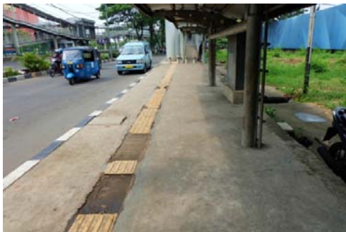
Fig 7. Poorly maintained guiding blocks in the side walks
