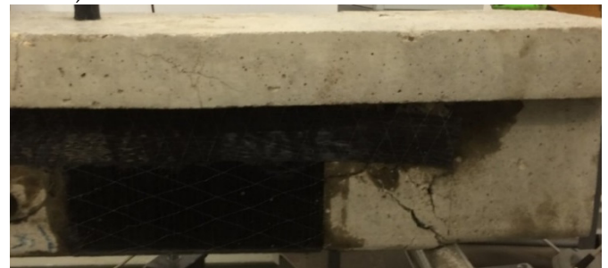
(c) S2-FRP1c (beam-end)
