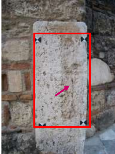
Figure App. I – 7: Crack 1, South Side (Metheniti, 2008)
