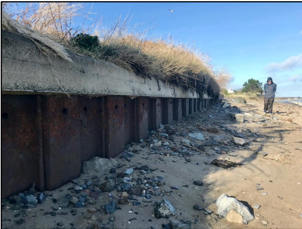
Figure 18: Evidence of the 1950s sheet pile located along the southern section of Burrow Beach.
