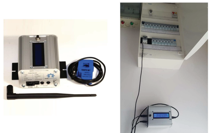
Fig. 1 EmonPi open-source monitoring device with clamp meter and WiFi antenna, and EmonPi installation at household mains supply.
