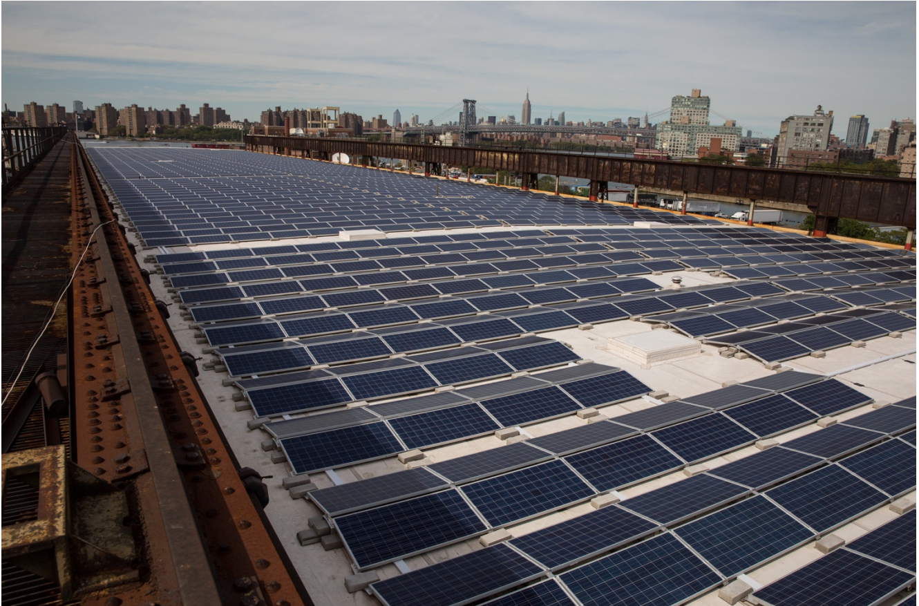
Figure 8: Largest solar installation in New York City located in the Brooklyn Navy Yard. Source: Brooklyn Navy Yard Development Corporation
