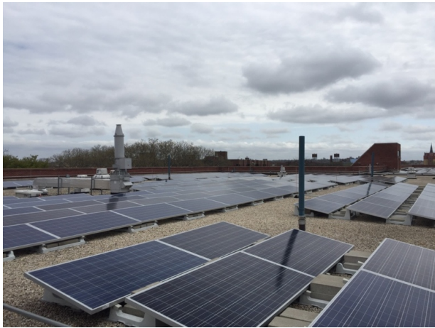
Figure 1: View of solar panels installed at Boys and Girls High School in Bedford Stuyvesant in Brooklyn.
