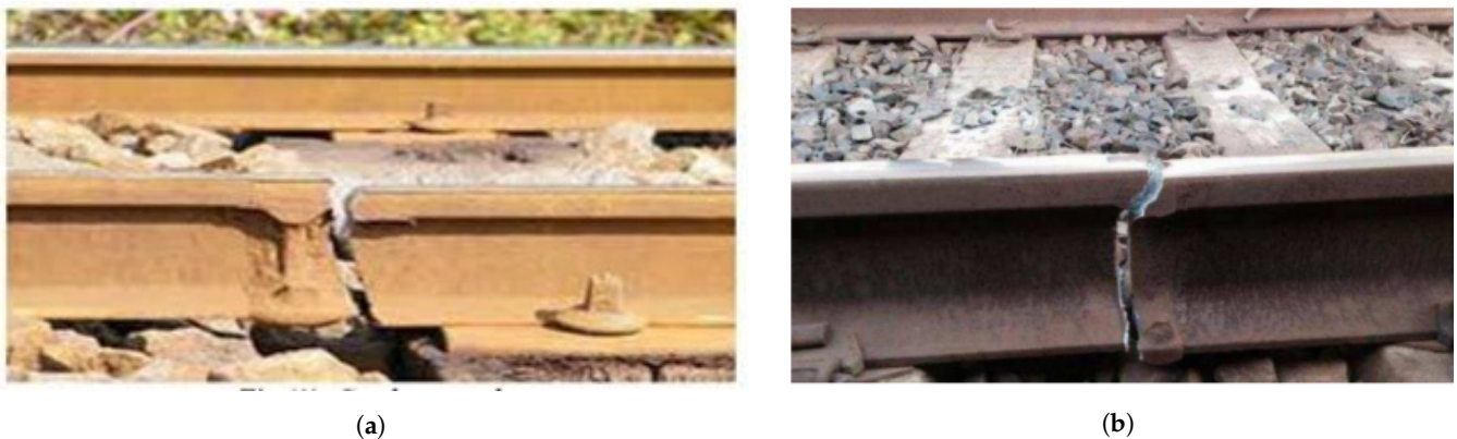
Figure 1. Samples of faults on railway tracks, (a) Destroyed patch [7]; (b) Partial crack [8]. Such faults can happen due to excessive loads, and the influence of cold and hot weather.
