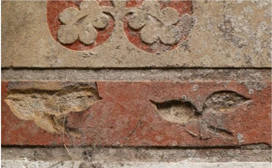
Fig. 62: Cottages, Down St Mary, Devon (c1875), attributed to Radford. Detail of main dado band, showing damage and lichen encrustation. Detail though and the overall effect remains bright and strong after 145 years.
