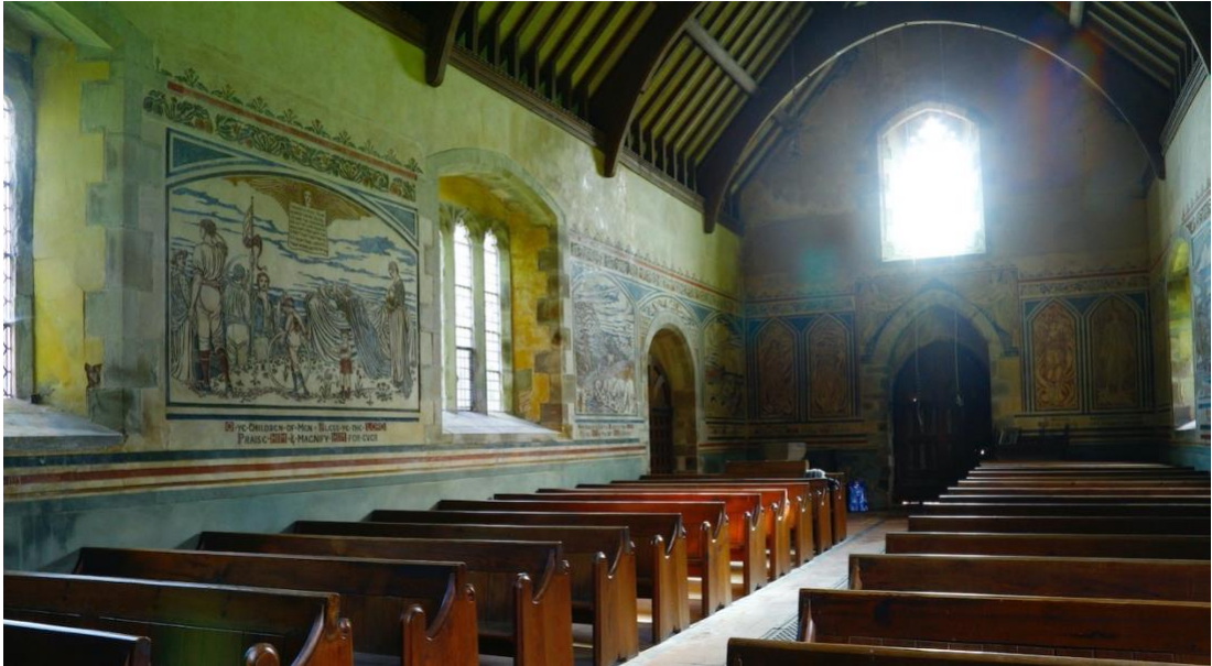
Fig. 9: St Mary the Virgin, Llanfair Kilgeddin, Monmouthshire (1888), by John Dando Sedding, architect, and Heywood Sumner, artist. South and west walls of nave showing the extent of Sumner's sgraffito.
