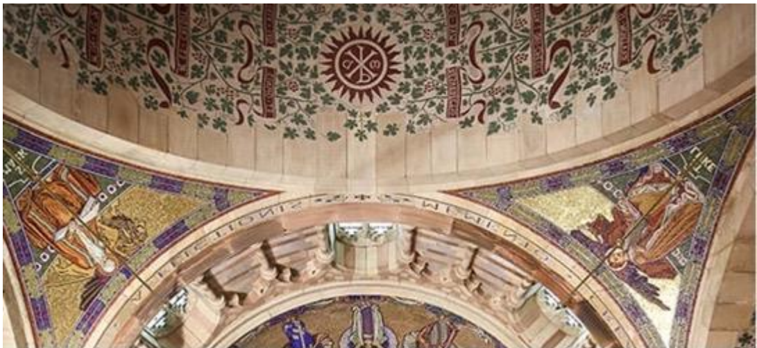
Fig. 3: Giggleswick School Chapel (1897 – 1901), by Thomas Graham Jackson. Section of dome and arched support with sgraffito leaves and grapes.
