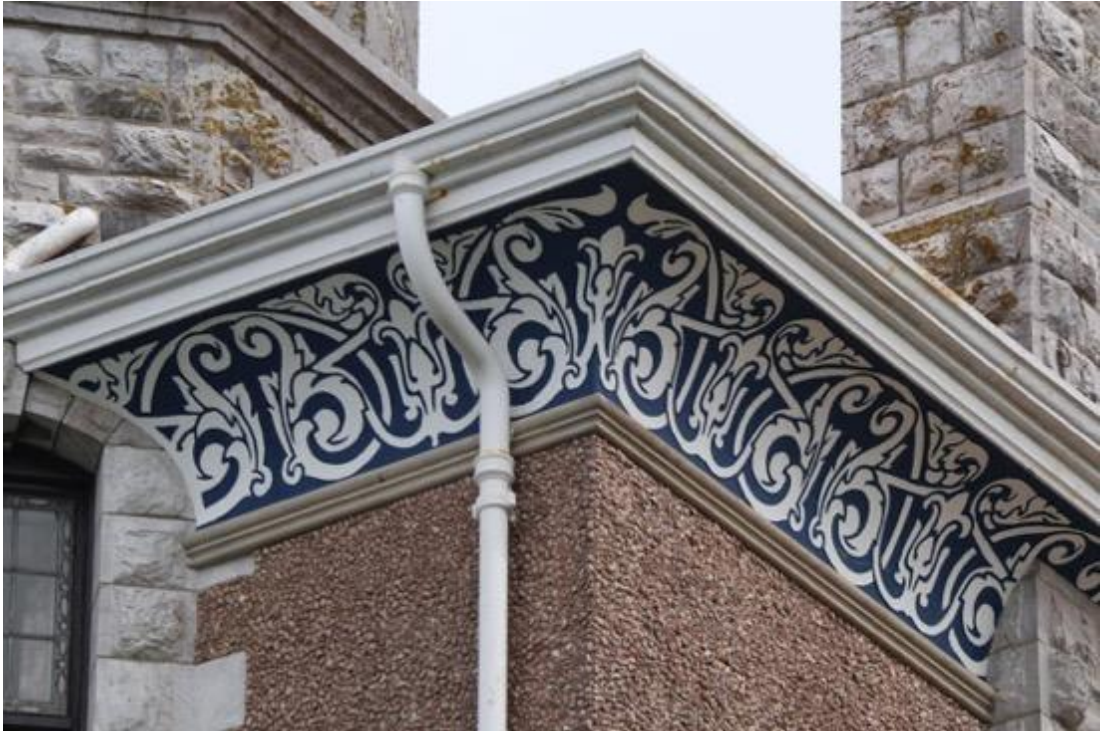
Fig. 12: Wolborough House, Brixham, Devon (1908), artist unknown. Detail of sgraffito on the heavily coved eaves, which is well protected from the weather.
