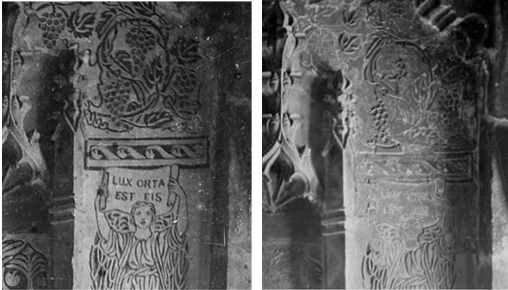
Fig. 5.1 and 2: Vicars' Close, Chapel, Wells (1886 – 87), by John Dando Sedding, architect, and Heywood Sumner, artist. View of east end of chapel. The damp affected sgraffito; left as completed before 1893, and right, showing severe signs of decay, sometime after 1893. 19
