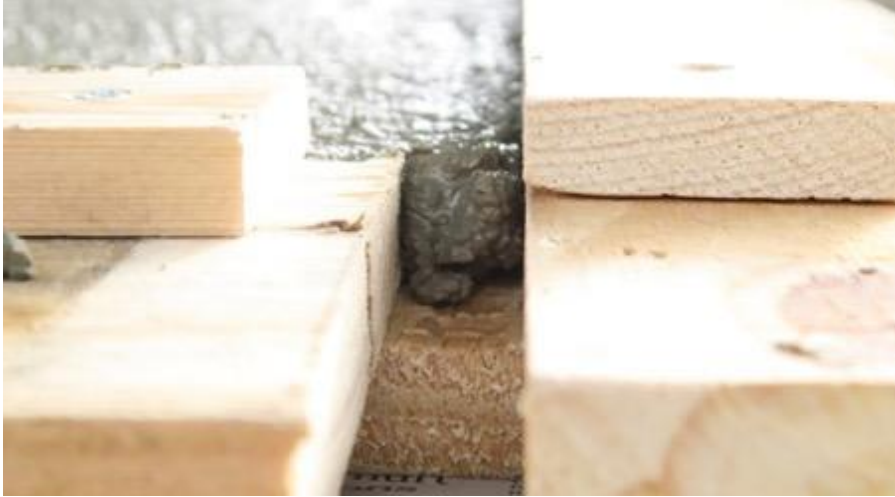
Fig. 6: Test panel 1. Base coat complete. View at gap in frame edges showing thickness and guide battens for depth of later coats.
