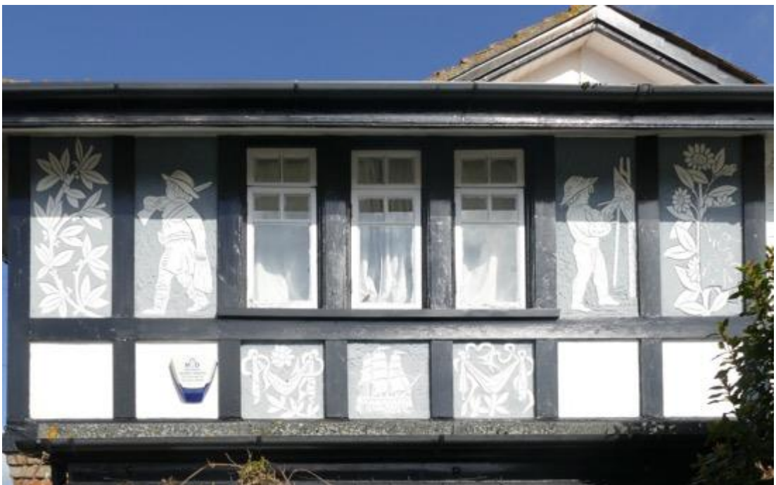
Fig. 58: 'Tresco', Birchington, Kent, by John Pollard Seddon (1882), architect, and George Frampton, artist. The depictions here appear clumsier, and even the three pretty panels below the window seem slightly awkward. Later overpainting will have accentuated this effect.
