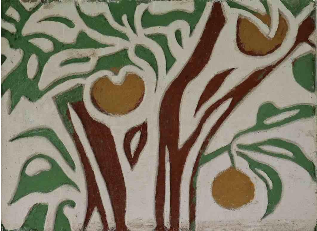
Fig. 28: Test panel 2, completed. Colour to cutting discrepancies very visible. Marks on the white surface have been cleaned off as far as possible without causing damage. Note repair – refixed dislodged piece at centre top-left, see also figure 30.
