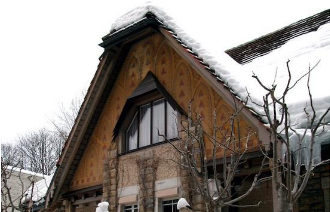
Fig. 7: Villa Fallet, La Chaux-de-Fonds Switzerland, (1904), by Charles-Edouard Jeanneret and colleagues. Sgraffito to gable.
