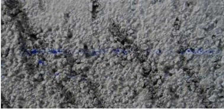
Fig. 8: Test panel 1. Detail of base layer surface with blue pounce line on roughened surface of the base layer.
