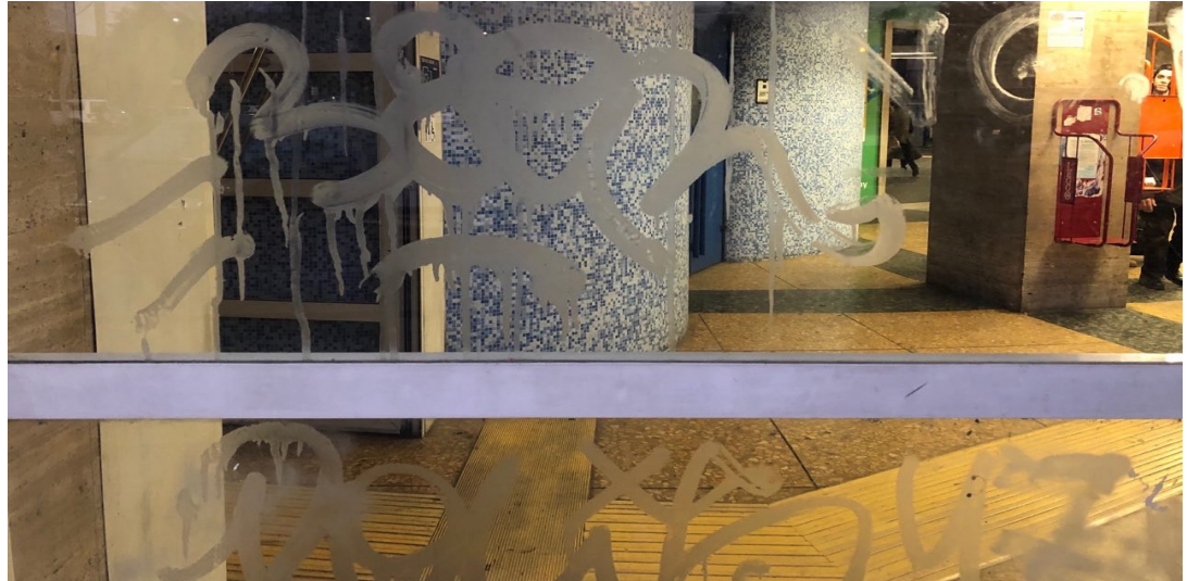
Figure 2-17. Destruction vandalism – Acid Etched Glass Graffiti, Piramide station, Rome. Photo by Mobasheri, S. (2019)
