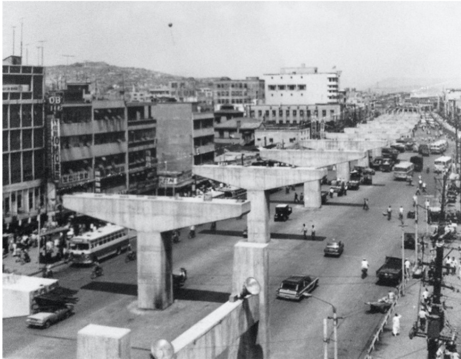
Figure 9. View of the Cheon Gye Cheon Expressway under construction in the early 1960s (Google Images).
