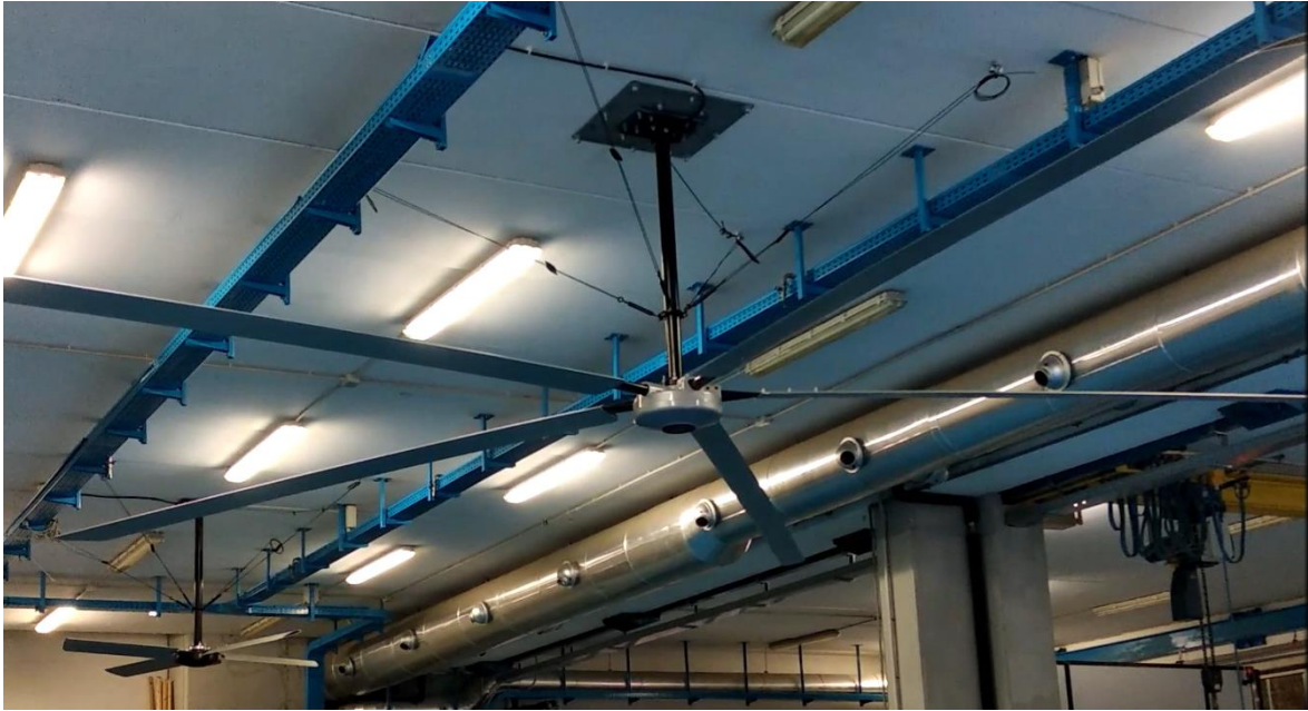
Fig. 44 Six meter diameter Fan supplied by Phase Motion Control inverter with RFO sensorless observer
