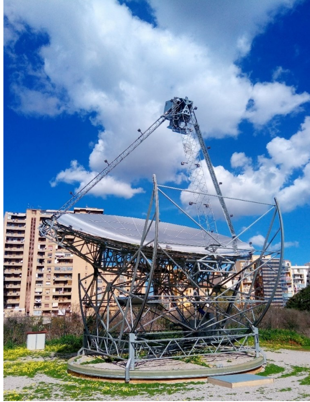
Figure 4: the dish-Stirling plant of Palermo
