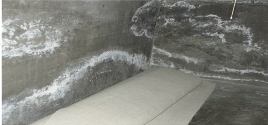
Figure 3. Excessive surface salt due to efflorescence phenomena.
