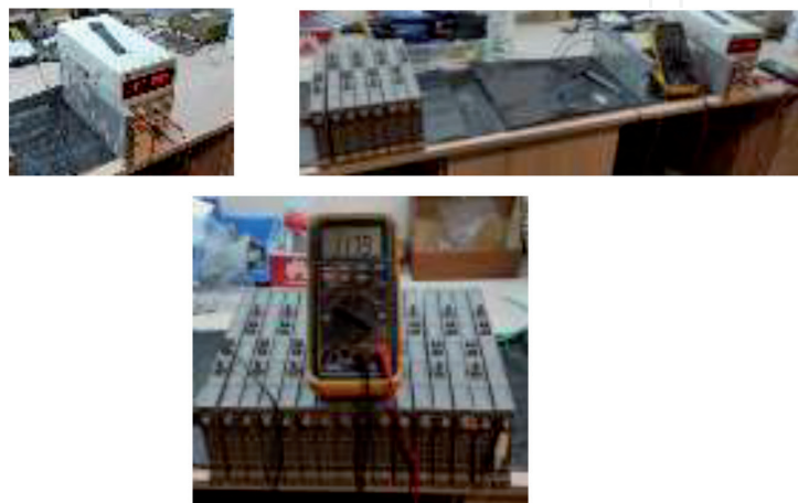
Figure 7. Reconfigured new battery packs.
