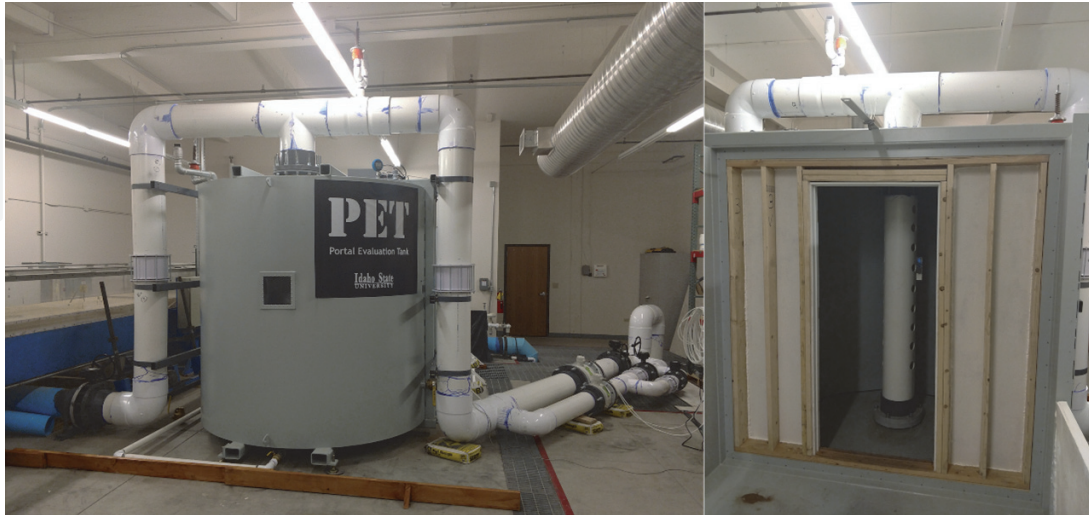
Figure 2. PET tank and piping.
