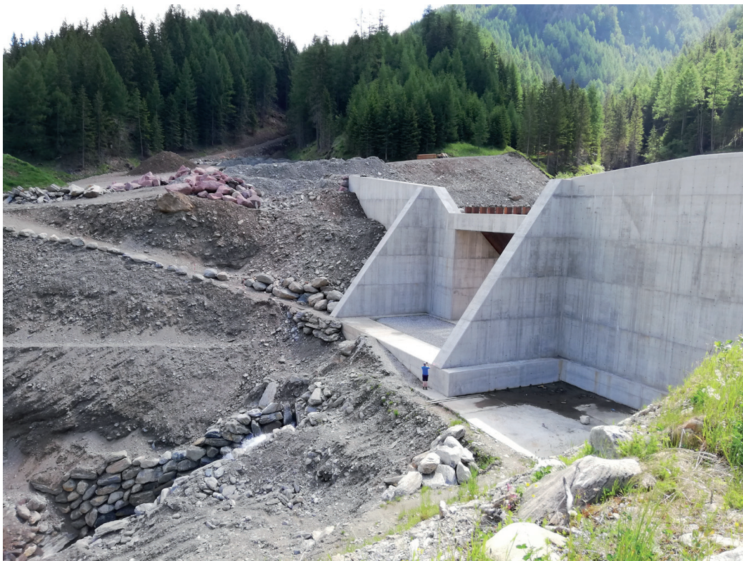
Figure 7. Technical measure against debris flows upstream of the buildings in Figure 6 . The site was visited during a GreenRisk4Alps field trip in June, 2019 (source: © S. Cocuccioni).
