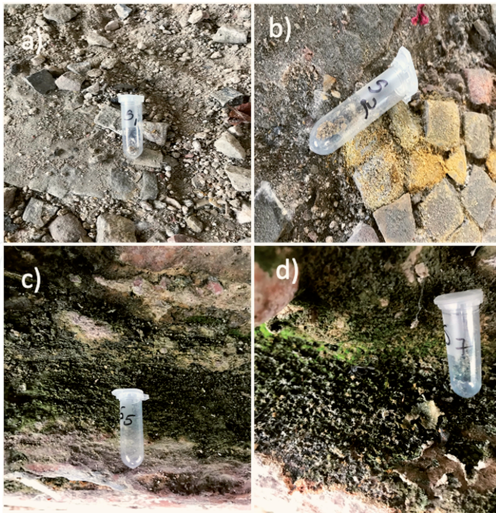
Figure 4. The affected areas of the mosaic by chromatic alteration and destructions (a, b), the biodegradation of wall surfaces (c, d).
