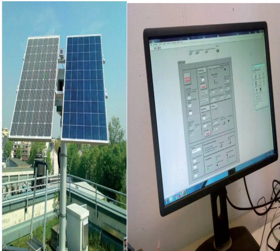
Figure 5. Solar tracking system at the Cologne University of Applied Sciences.
