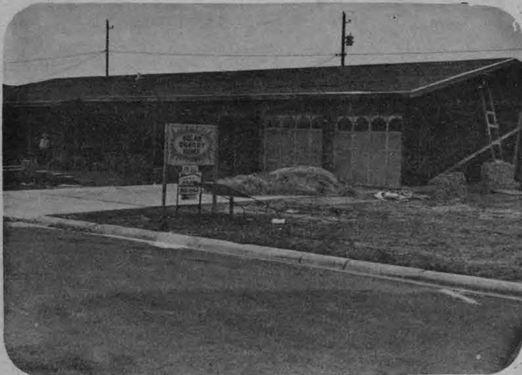
SOLAR ENERGY HOME -- Under construction just off S. Sugar Rd. is what may be the Valley's debut into solar energy homes.
