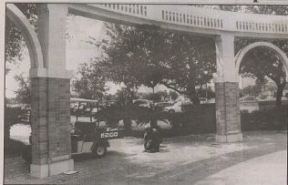
Rogelio Rodriguez fixes bricks under the arch in front of the library after the center column was removed.
