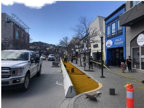
Fig.19: Execution of Sidewalks extension Kaisar, V. (2021, June 15). B.C. government in favour of municipalities making temporary patios permanent in post-pandemic world. Radio NL - Kamloops News.
