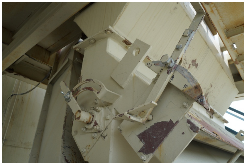
Figure 29. Primary and Secondary air inlet valve adjustment system for one of the AC22.5GI air-classifiers at LuckStone’s Goose Creek plant
