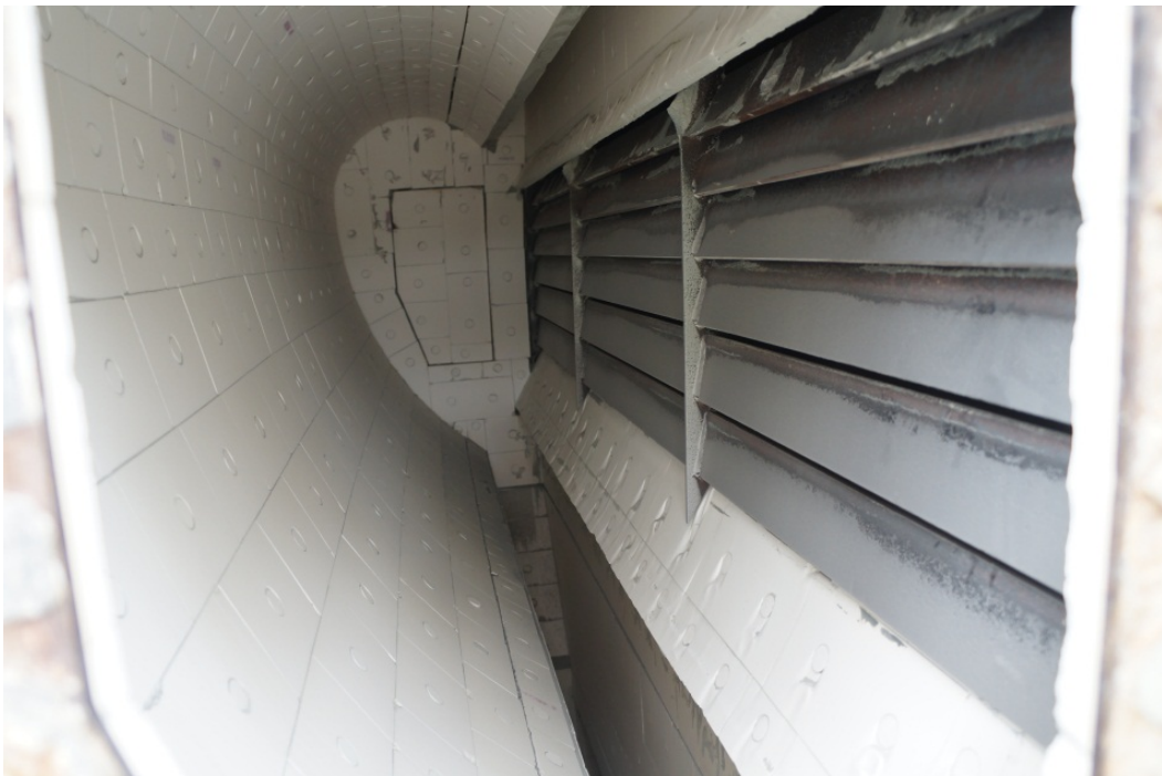
Figure 26. Ceramic linings and vanes inside one of the GI classifier units in Figure 2, after 8 years of operation the wear of the linings is still negligible
