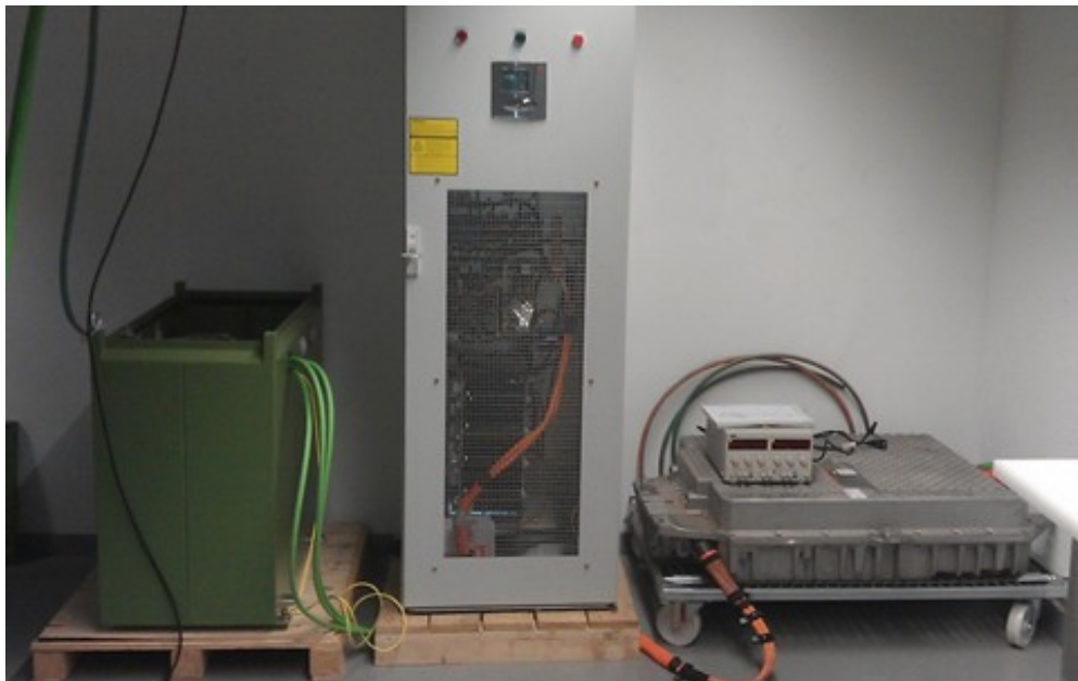
Figure 11: Second-life battery set-up
