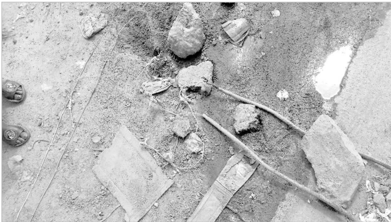
Figure 8: Illegal electricity connections on the floor of a dwelling in Amalinda.
