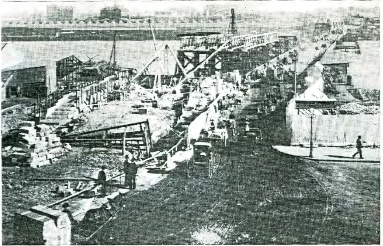
The New Pymont Bridge Under Construction Alongside The Old Bridge, 1900. Source, DMR Archives
