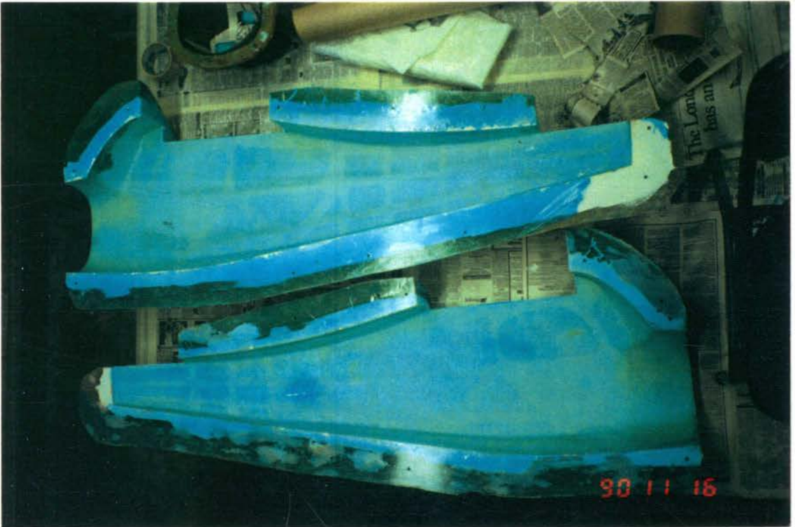
Figure B.37 One complete layer of ACI225 split strand fiberglass cloth applied with epoxy resins, and a second layer along load-lines.
