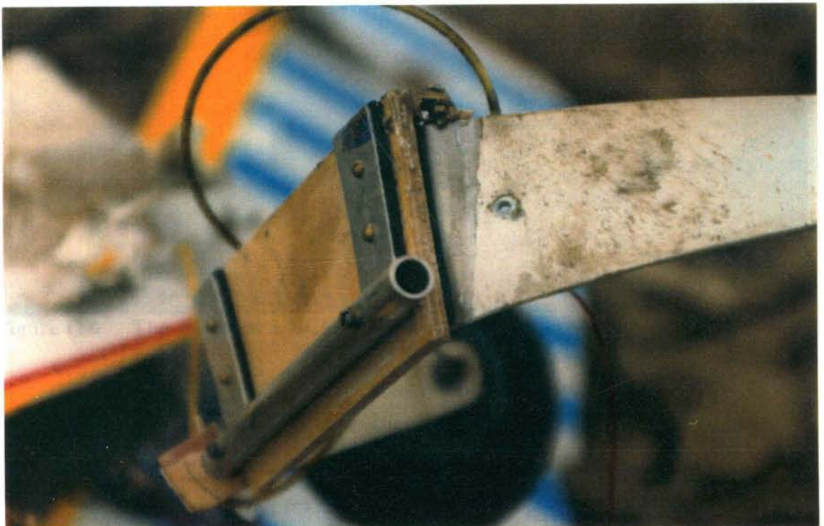
Figure C.5 Shows the failed strut fitting attachment point.
