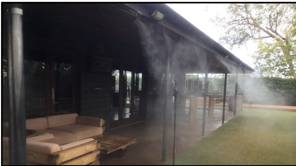
Figure 1.2 Water mist system in operation
