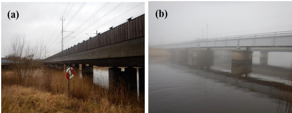
Figure 8. Pictures of (a) Skälderviksbron and (b) Flygarebron located in Rönne å where local scour has been observed (from BaTMan, 2021)
