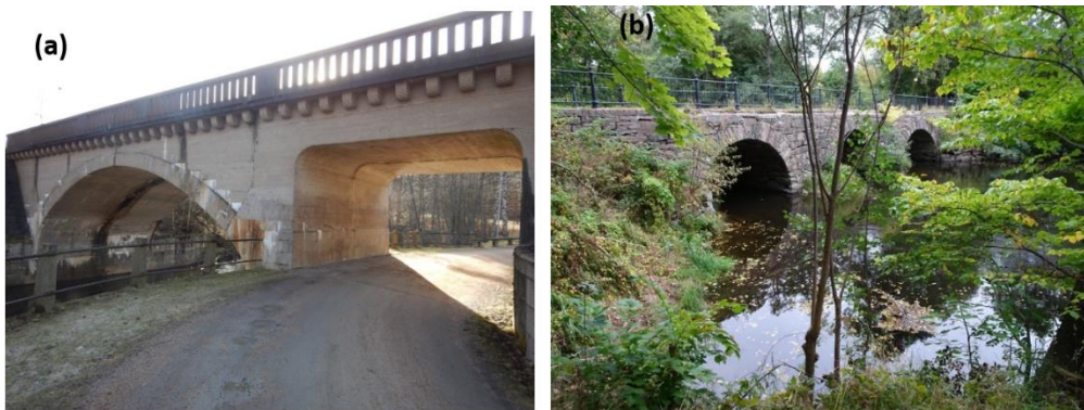
Figure 10. Pictures of (a) Järnvägsbron (across Sävån) and (b) Wamme bro located in the Sävån where local scour has been observed (from BaTMan, 2021)
