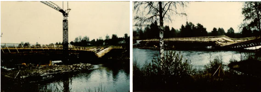
Figure 16. Failure of the bridge over Österdal River during construction due to scour around one of the piers (from Dargahi, 1982)
