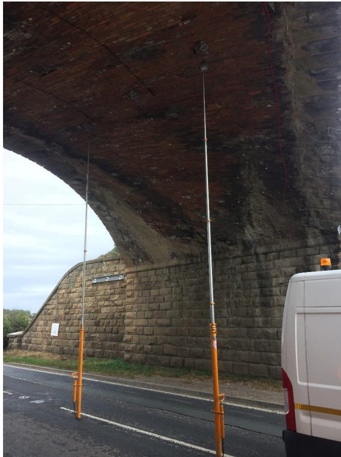
Figure 4.4: View of deflection pole monitoring at CFM-5, with poles installed underneath both rail tracks (after Thompson et al., 2019)
