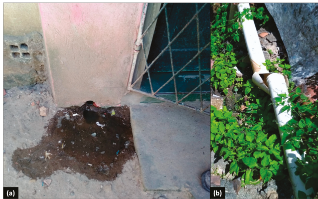
Figure 16. (a) Presence of water on the slope surface; (b) Damaged drain pipe.
