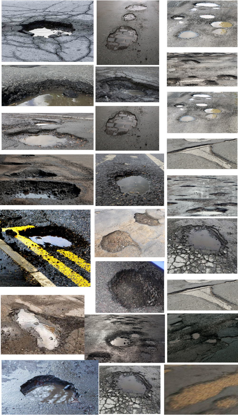
Figure 37 : Damaged road surface (DM02)
