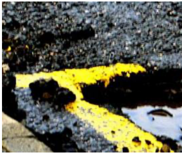
figure 40: A pothole image to be augmented
