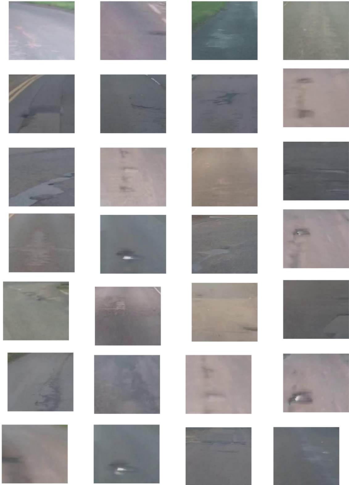
Figure 36: Damaged road surface (DM01)
