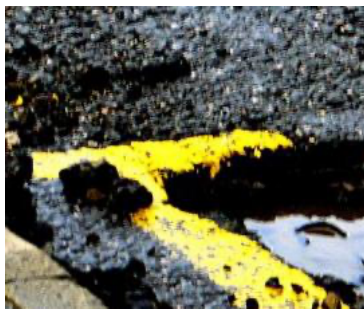
Figure 38: A pothole image to be augmented
