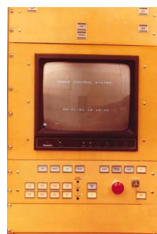
Fig. 19. EMACK control panel.
