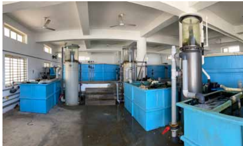
Units of the 30 tonne Recirculating aquaculture systems
