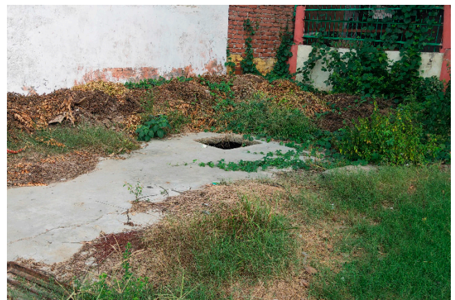
Tikonia Park, Nirla Nagar, Lucknow: open manhole
