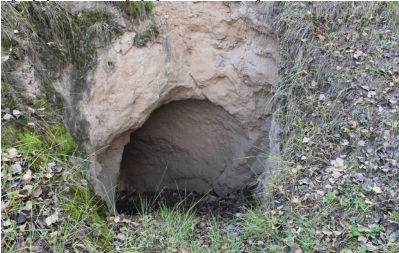
FIG 13. A hole made in the castle wall by invaders during the Qing Dynasty in order to attack the Sughua people chansi , and villages' purghan (7 October 2013, Jugui).
