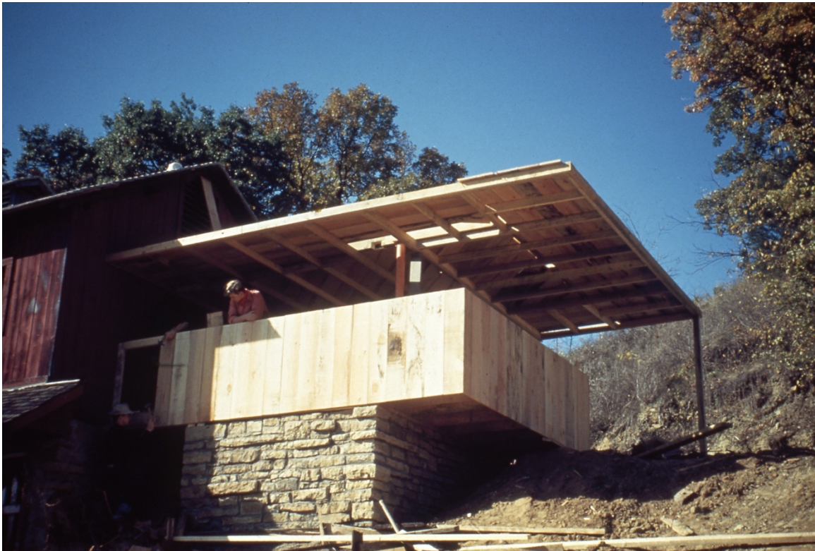
Figure 13: Balcony addition to the apartment above the calf pen under construction, c 1940-50. Photography by Loid Davidson Gottlieb. Courtesy of Taliesin Preservation Inc.
