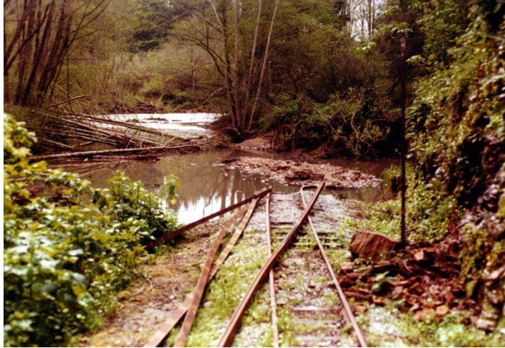
Figure 6 - Picture of Washout from 2017, from SPRR Facebook
