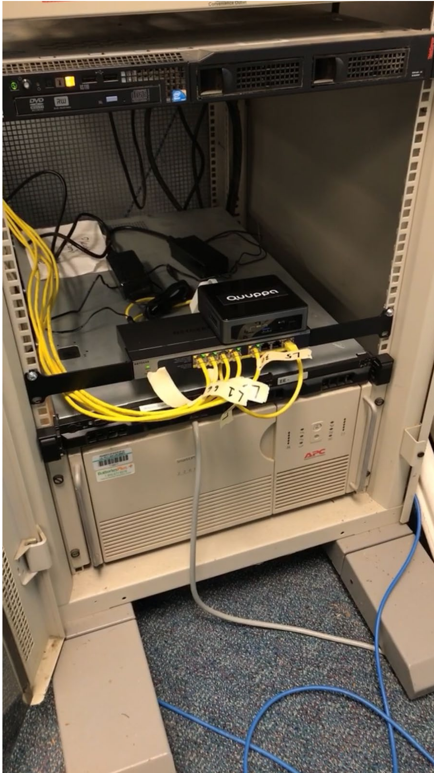
Figure 10: QPE server and PoE switch installed in server rack
