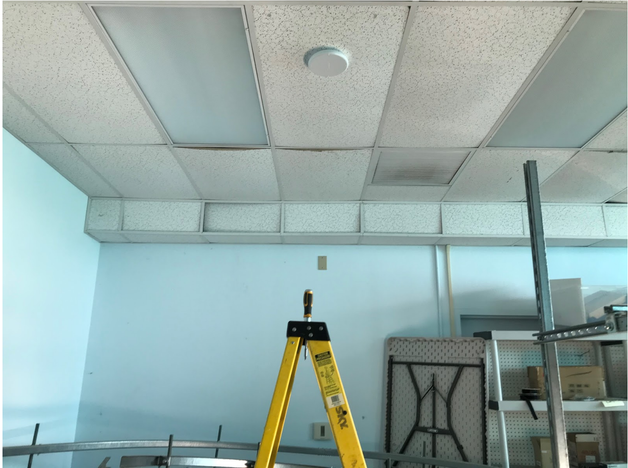
Figure 9: Quuppa Locator installed in PolyGAIT ceiling
