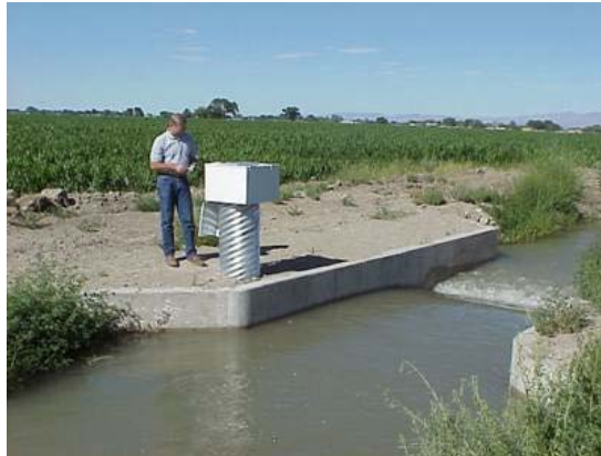
Figure 3. Concrete broad-crested weir built in a rectangular cross-section (Truckee Carson ID)
