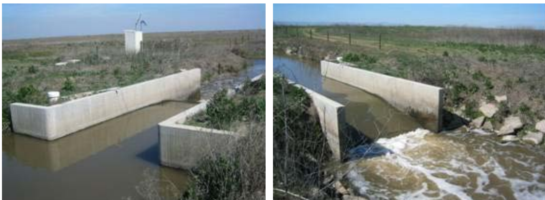
Figure 4. Concrete Replogle flume in the Hollow Tree Drain (Grassland Water District)
