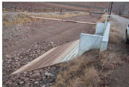
Figure 9. Punch plate at the inlet to an irrigation district lateral pipeline. 1 inch holes, 50% open area, to maintain less than 0.5 ft/sec through the holes (0.25 ft/sec approach velocity).
