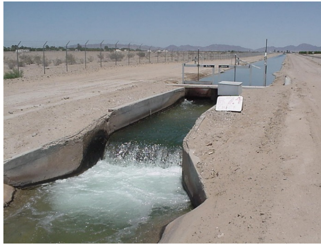
Figure 43. Example of a suppressed weir. The upstream channel has the same width as the weir crest. In this particular case, the walls diverge immediately downstream of the weir, so the nappe is aerated.
