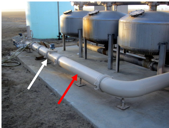
Figure 3. A propeller meter (white arrow) installed downstream of drip system filters, with a long, straight pipe section upstream of the meter (red arrow)
