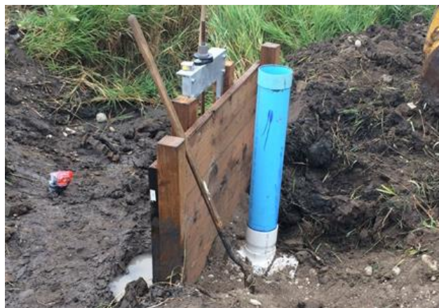
Figure 19. Stilling well installed on metergate with proper diameter, position, and height but not precast.
