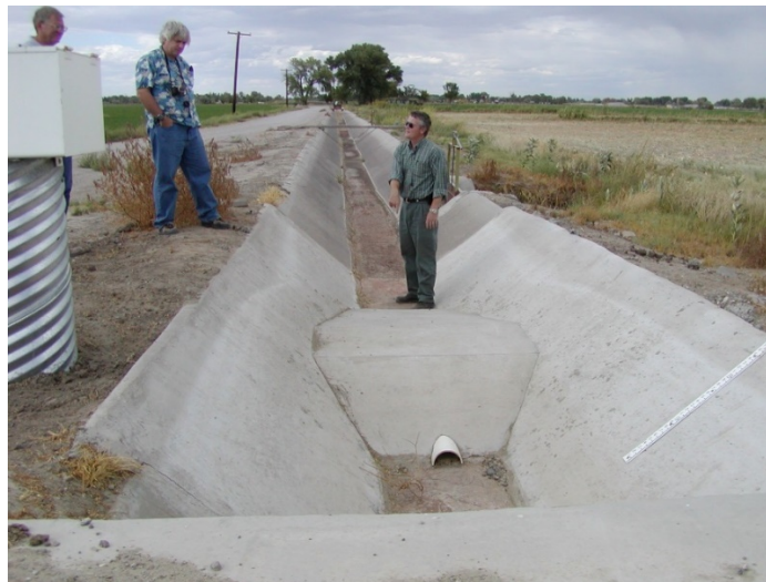
Figure 38. A "Replogle flume" installed on a ditch with high flows in Truckee-Carson ID in Nevada. This is constructed in a trapezoidal section of canal.
