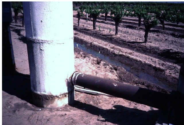
Figure 47. The discharge pressure of the pump will change over time with this type of direct connection to a standpipe
