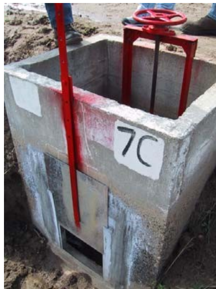
Figure 28. Alta ID rectangular orifice gate (front) provides flow measurement, while sluice gate (rear) provides flow control
