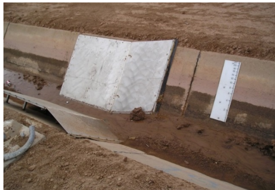
Figure 46. Flat-bottomed (actually, a “Vee” in this case) flume immediately after construction. The sediment will flush out once water flows in the ditch.
