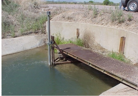
Figure 8. Open propeller meter installed at the discharge end of a large full turnout pipe. Water flows from right to left
