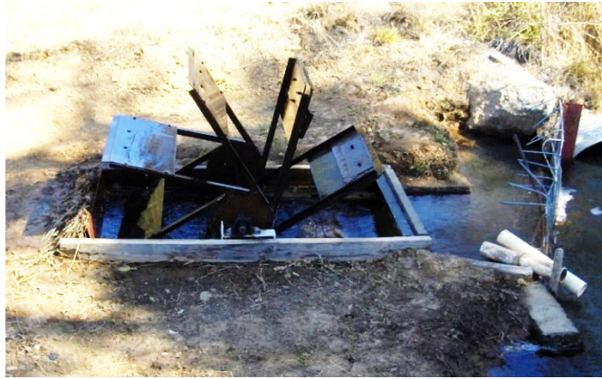
Figure 10. Locally fabricated trash screen in Browns Valley ID
