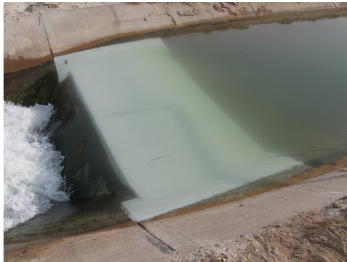
Figure 40. A flume with an ePaint™ coating to minimize algae growth
