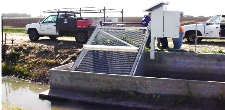
Figure 11. Automatic screen upstream of a turnout in Merced ID. Note the wall that helps prevent sand from entering the turnout.
