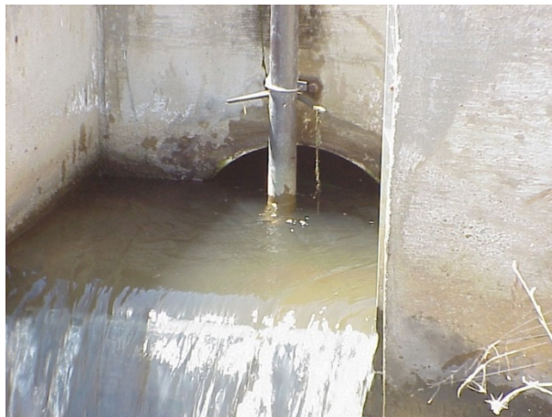
Figure 7. Weir boards are installed downstream of an open propeller meter. Obviously, these are not high enough to create a full pipe condition.
