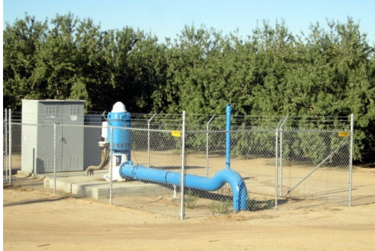
Figure 5. A loop in a pipe is installed to keep the upstream pipe section full. A continuous acting air vent is needed at the top of the loop.
