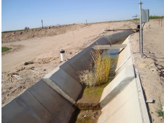
Figure 39. Flume with expensive monitoring and a slight maintenance problem
