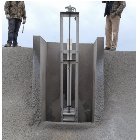
Figure 24. Installed pre-fabricated canal metergate (Fresno ID, 2019)
