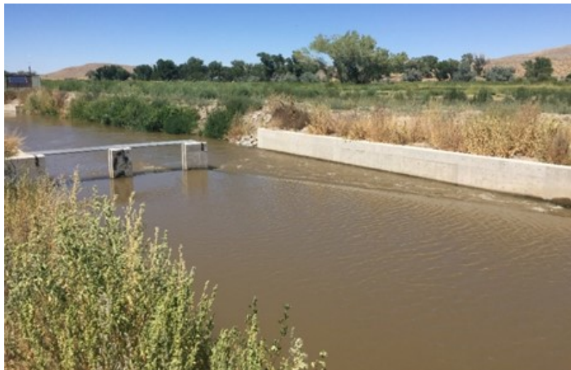
Figure 12. Settling basin and sediment wall on Fox Mickey Canal
