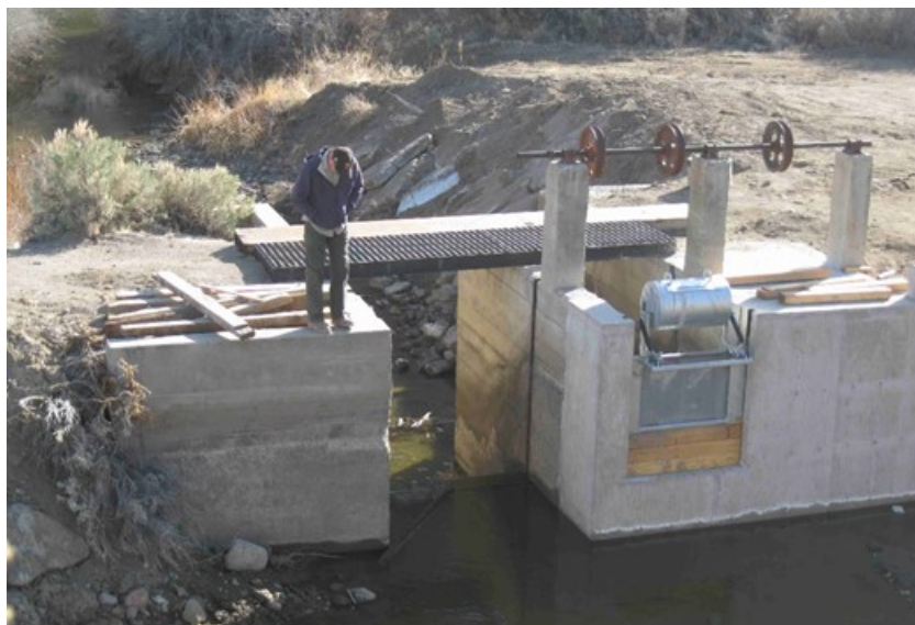
Figure 9. Flap gate installed in the Saroni Canal
