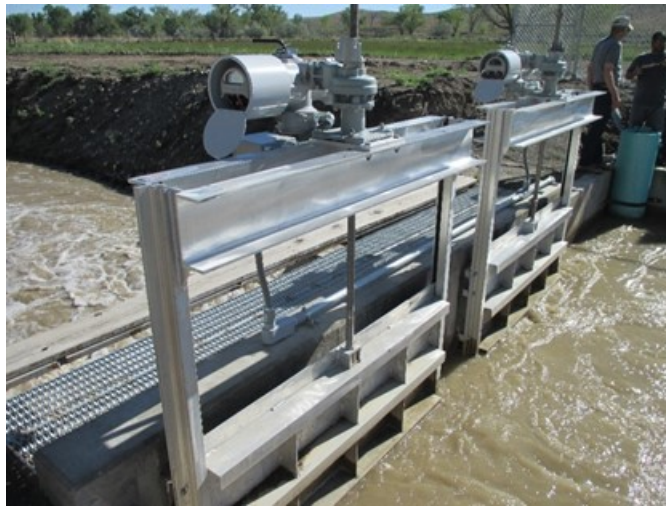
Figure 13. Automated gates on Fox Mickey Canal
