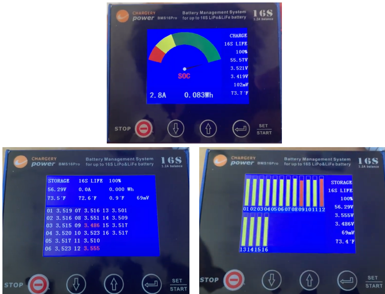
FIGURE VII CHARGERY BMS16T100 SCREEN READ-OUTS FOR THE SYSTEM.
