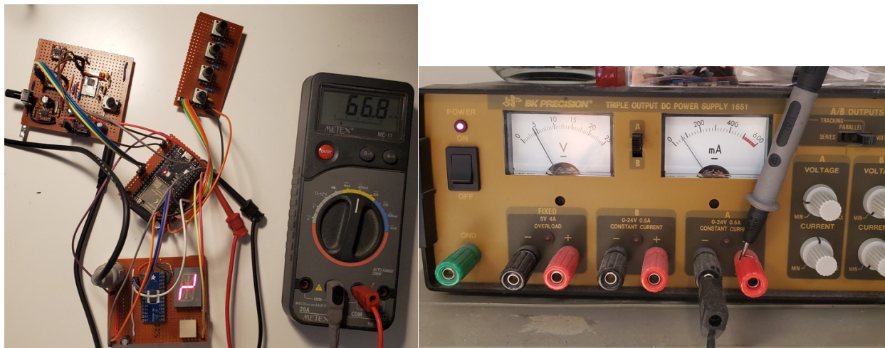
FIGURE 36: BATTERY POWER DRAW TESTING
