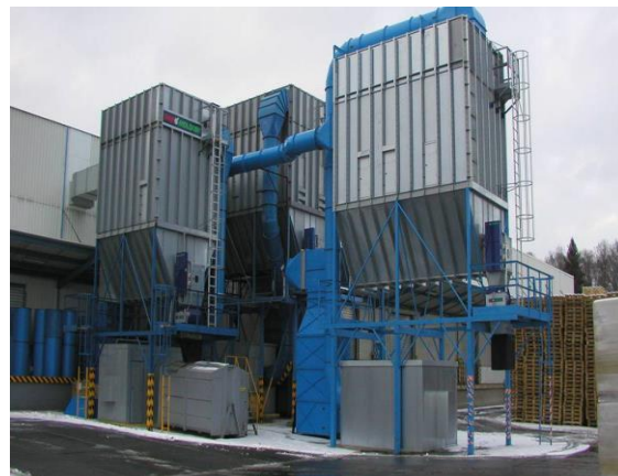
Small Dust Handling Facility
